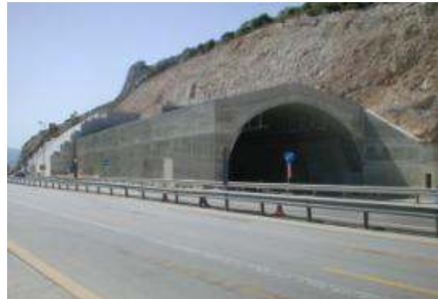
AS1 tunnel entrance portal structure / cut & cover (Highway PATHE, Kakia Skala section)
