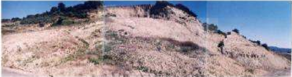
Existing failure of the open cuts with material removal inside the road traffic sidewalk outline
