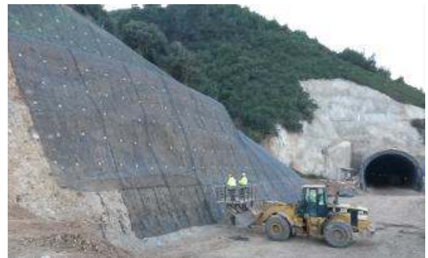
High open cut with fully bonded permanent anchors and appropriate slope protection with anchored wire mesh
