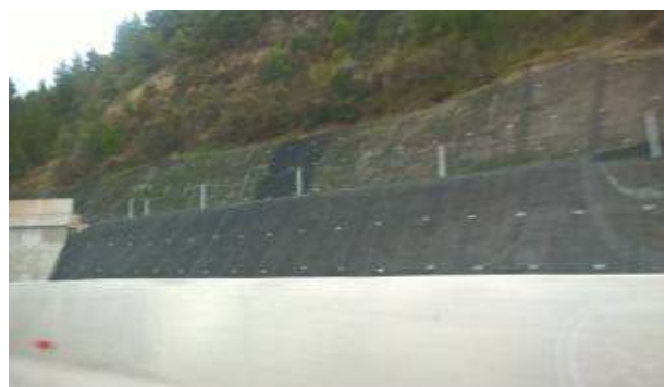
Open cut with fully bonded permanent anchors and appropriate slope protection with anchored wire mesh and rock fall protection barrier
