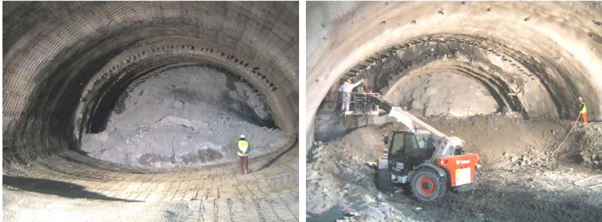
Figure 7. Tunnel T2 - Stiffening Inner shotcrete shell in top heading – “Short pilot tunnel” application
