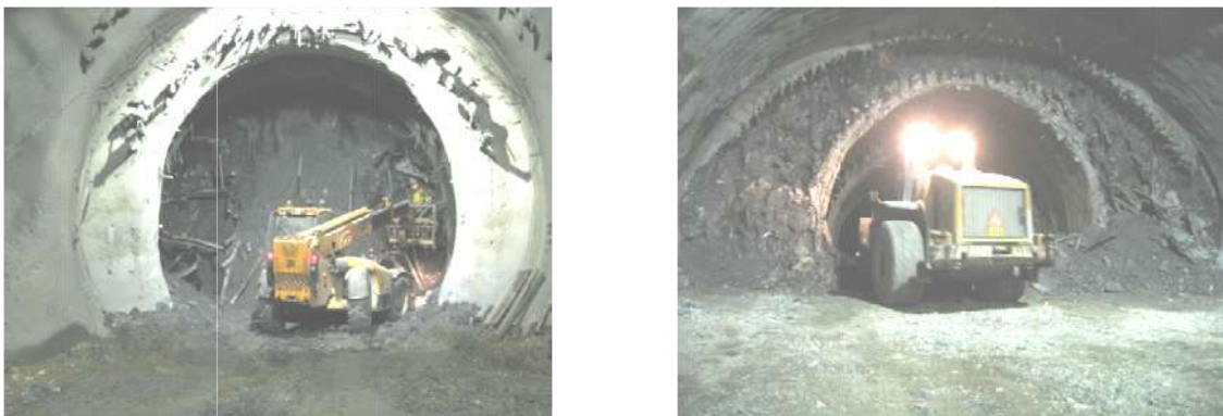
Figure 3. Tunnel T3 – Rehabilitation Works at ch.12+400 – a. pilot tunnel phase; b. widening phase
