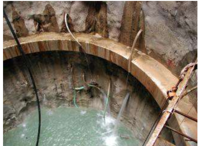
Figure 5. Water inflow from drainage holes in the shaft.
