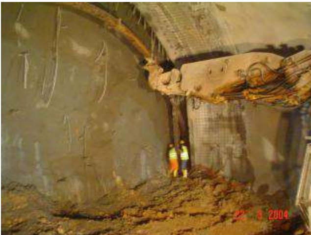
Figure 6. Top heading excavation of the Station tunnel. Installation of the HEB 180 steel arches.
