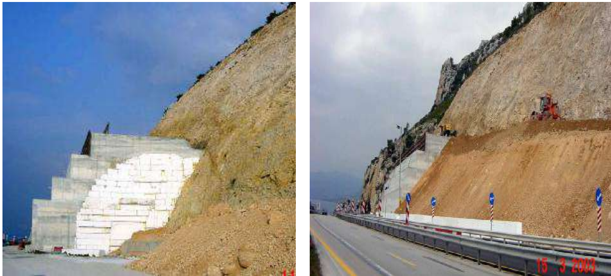
Figure 3 Reinforced concrete structure in east portal of right bore of AS1 with polysterine.
