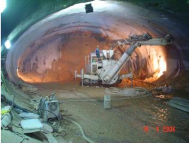
Figure 5. Installation of the forepoling tubes at the top heading of the Station tunnel.
